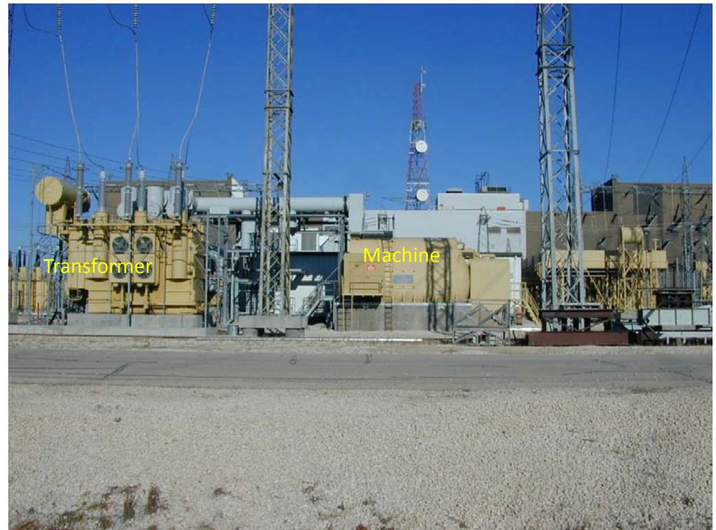
Dorsey Synchronous Condensers
