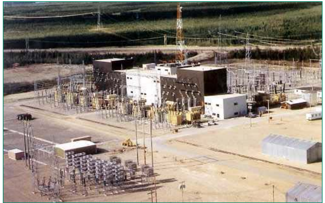
Converter Station (Henday)
