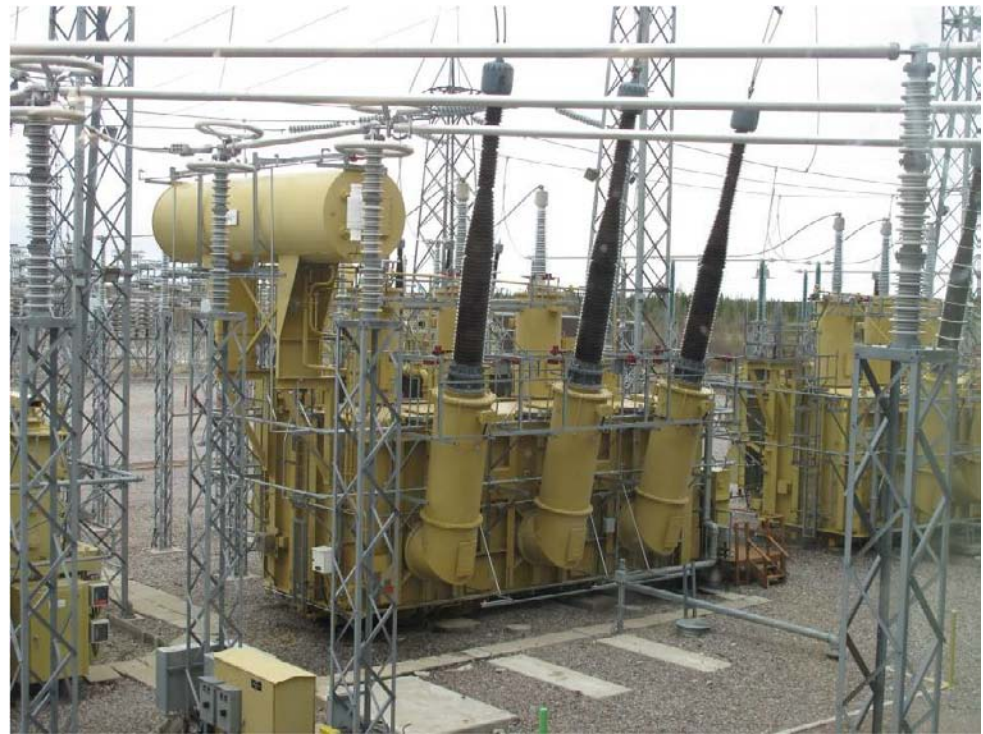
BPII Converter Transformers
