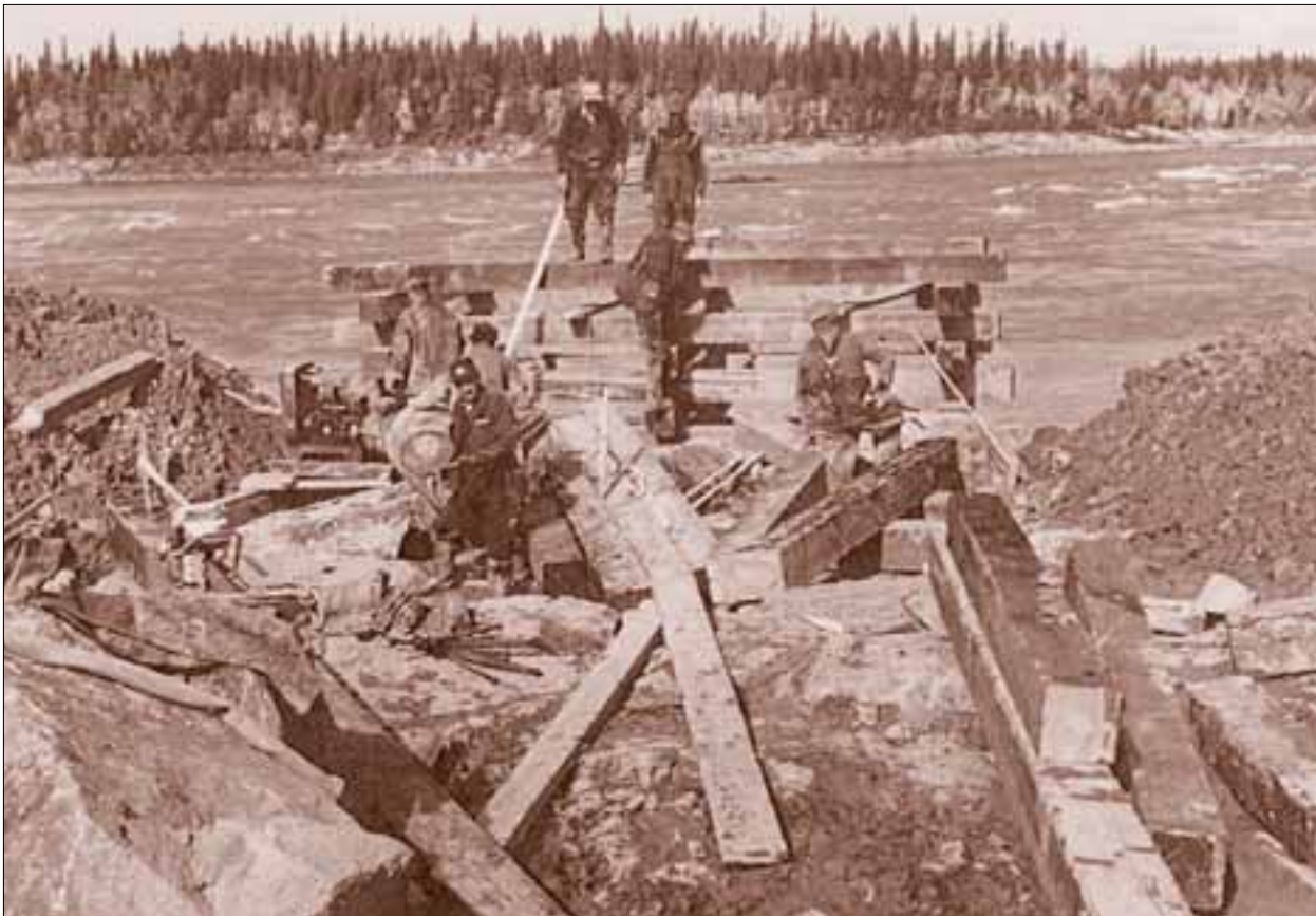
Start of the dock construction at Kelsey from which scows would carry material across the river. September 1957.
