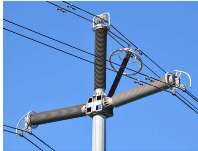
Tower top of 420 kV tubular line in Norway
