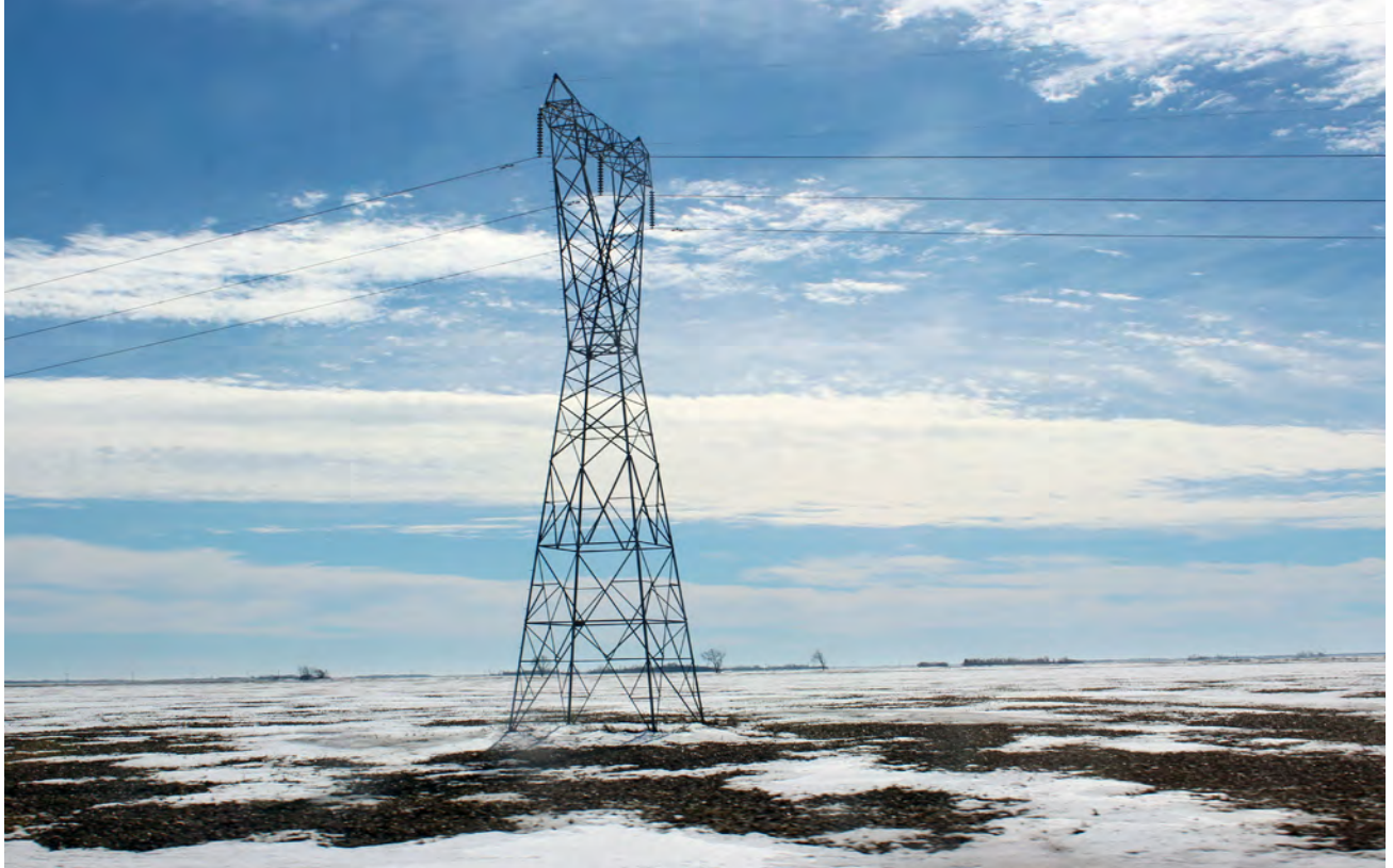
Guyed Lattice Steel Structure (Photo: Olivia Mancuso)
