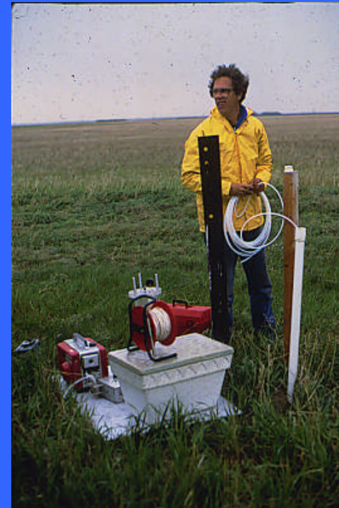
Narrow diameter monitor well, also called piezometer
